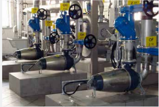
Fig. 3 Grundfos sewage pumps on individual foundations.
