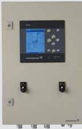
Fig. 22 Dedicated Controls control cabinet
